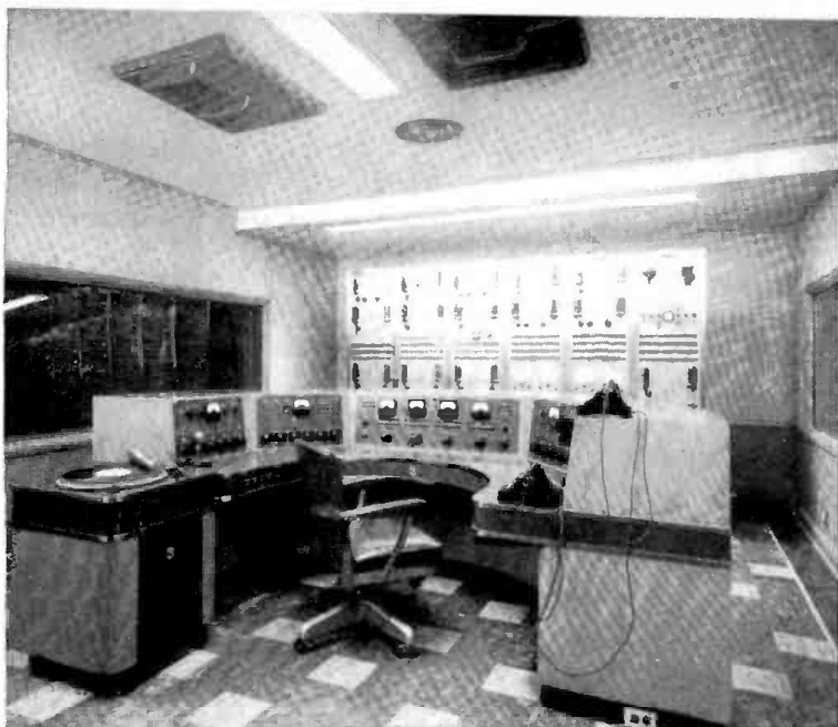
WISH, Indianapolis. This master control desk with 6 de-luxe audio equipment racks (in-line), visible at rear, is only a part of WISH's 4-studio installation—custom-built by RCA. It provides complete push-button control (independent or simultaneous) for 4 program channels. Five master desk panels, left to right: Studio "A" control, MCR-NET-REM control, master monitoring and switching, Studio "B" control, and Studio "C" control.
